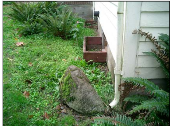
Grade toward foundation
